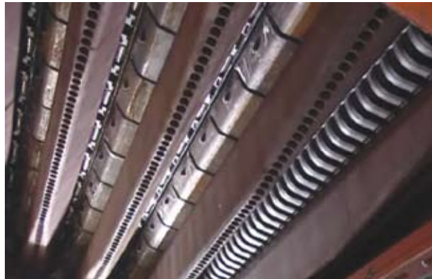
Below the grate: No flex tubes below the grate
