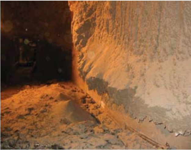
Slag deposits over the grate
