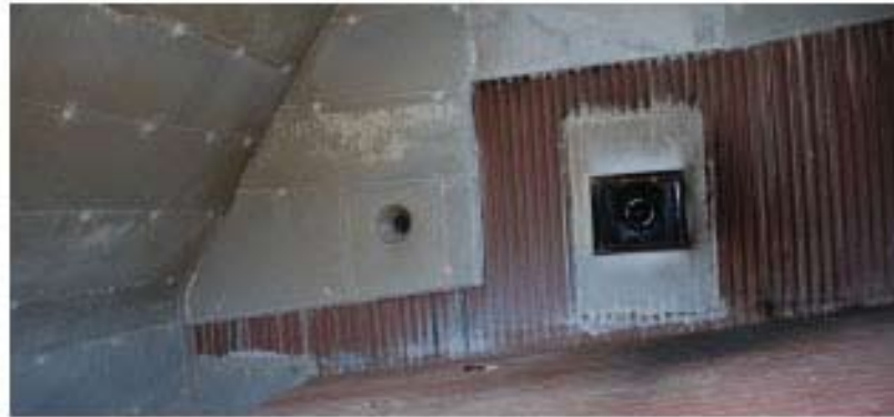
The combustion chamber
