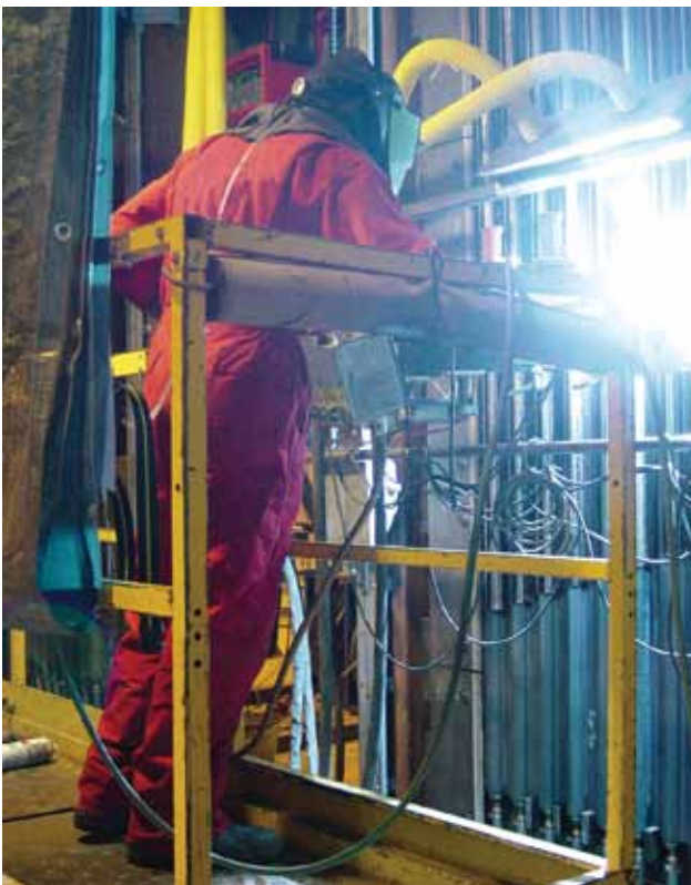
Our certified welders and fitters carry out high-quality work and are available 24 hours a day.
