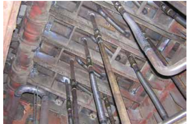
Tube work at the Häsleholm plant. The water system beneath the grate consists of steel pipes with steel flex connections
